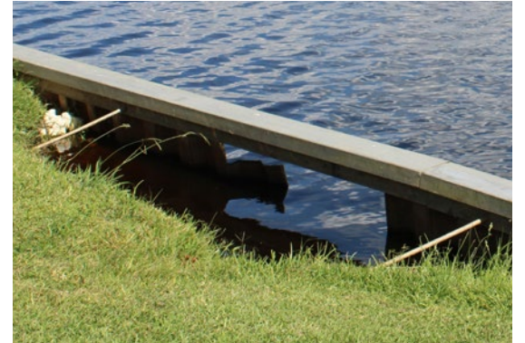
The Pasquotank River is eating away at the bulkhead and eroding the soil, causing many holes along what appears to be a pristine waterfront – from a distance.
